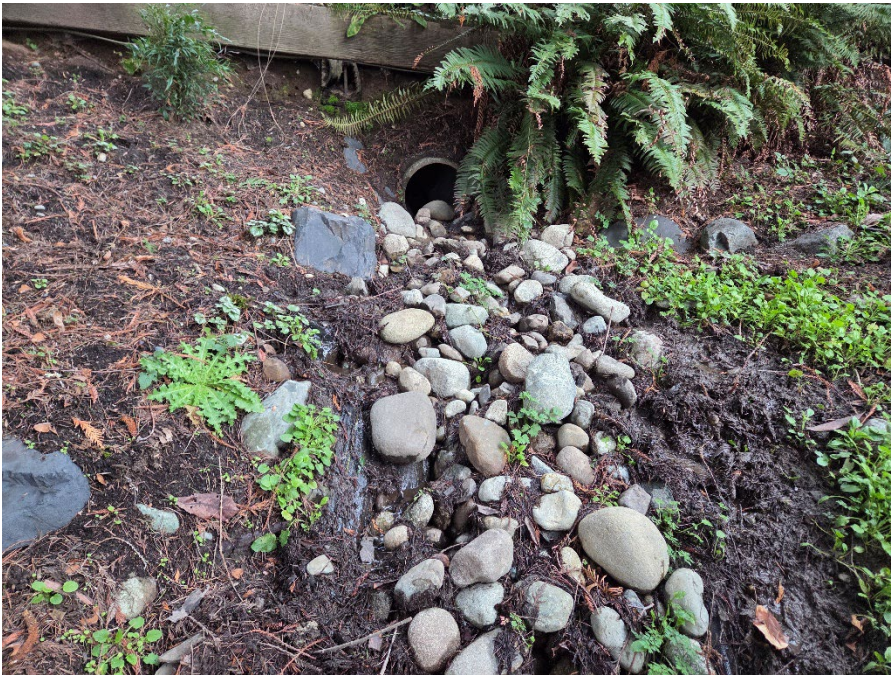
Photo 10. Piped stormwater outfall onto open channel lined with black fabric and cobble with no distinct scour or bank.
