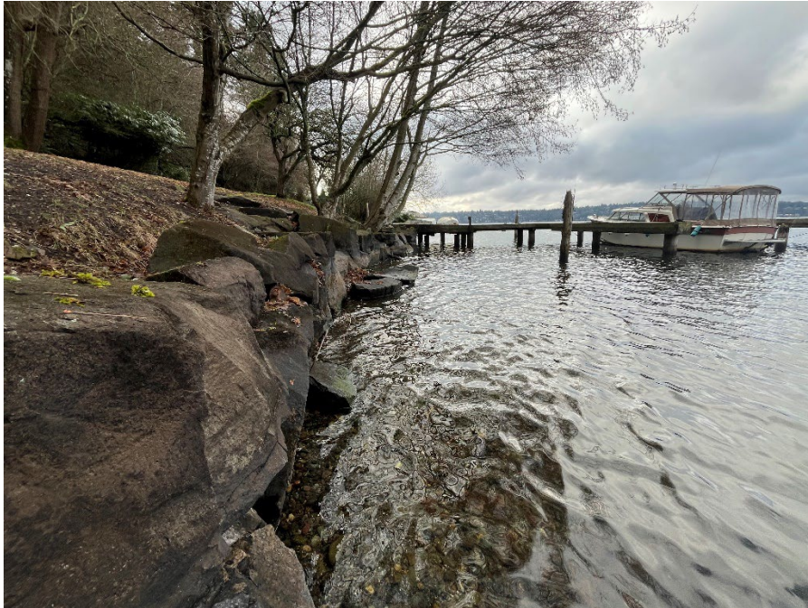
Photo 3. View looking south at the bulkhead from the northern corner of the project area.
