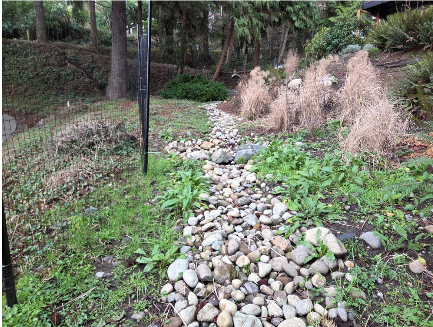
Photo 11. Open channel lined with black fabric and cobble with no distinct scour or bank.
