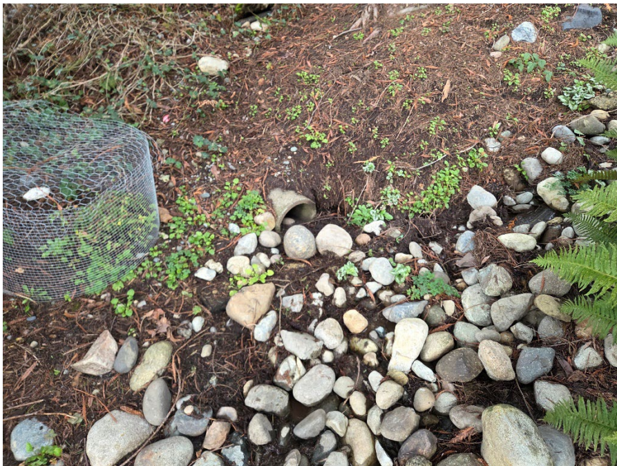
Photo 12. Piped stormwater outfall onto open channel lined with black fabric and cobble with no distinct scour or bank.
